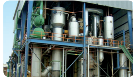
Preparation and extraction plant IASA – Bolivia 1.500 t/d
