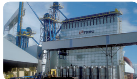
Reception Installation Agreco Alto Araguaia/MT 300 t/h soybean
